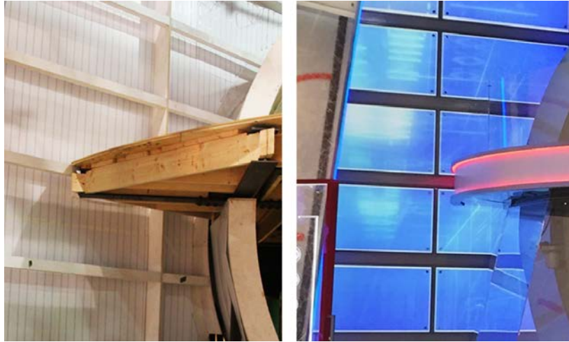
White LED tape installed vertically (L) to backlight blue, frosted Plexi (R)
